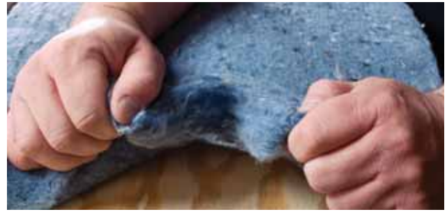
Tear with your hands lengthwise! Cotton Armor's easy fit around common obstacles found in wall cavities reduces acoustical shortcuts.
